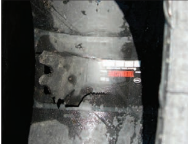
EFFECT: Improper Repair or Improper Repair Procedures CAUSE: Premature Failure of Repair
