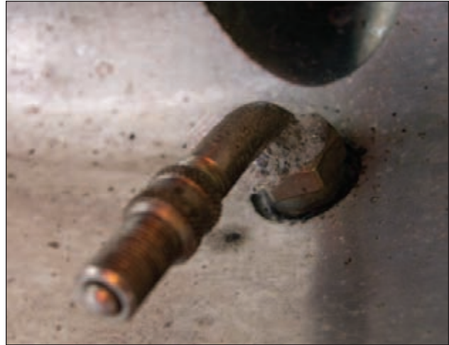
EFFECT: Leaking Valve, Grommet, or Wheel CAUSE: Improper Installation - Torque, Lubrication, Corrosion
