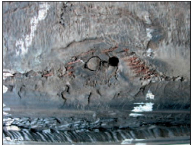
EFFECT: Missed Nail Hole CAUSE: Repaired from the Outside Resulting in Missed Damage
